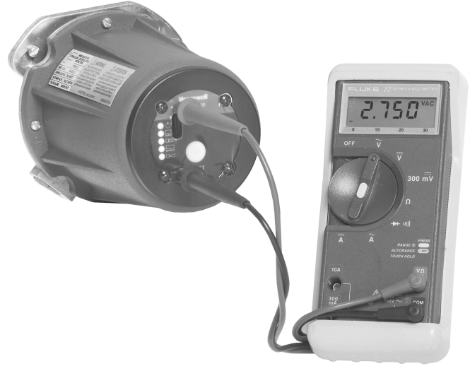
Fig. 5. Measuring the flame signal voltage.
