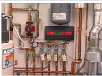
Ditter Heating and Cooling, Minnesota
