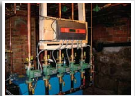
Downeast Energy, Maine
