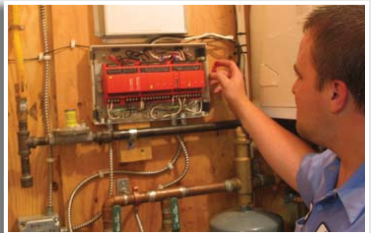
Palo Heating, Cooling & Plumbing
