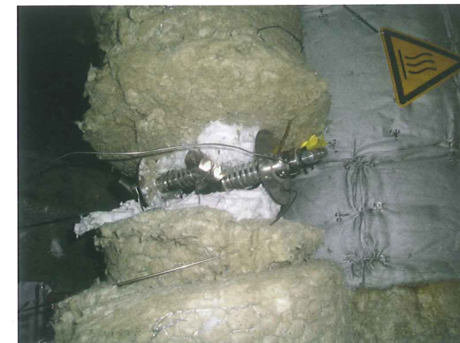
AS-Schneider dual shut-off valve installed in COMTES700 for a long-term design test at 700 °C (insulation removed)
