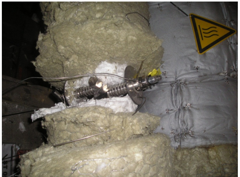
Fig. 1: AS-Schneider dual shut-off valve installed in a test plant COMTES700 for a long-term design test at 700 °C (insulation removed)
